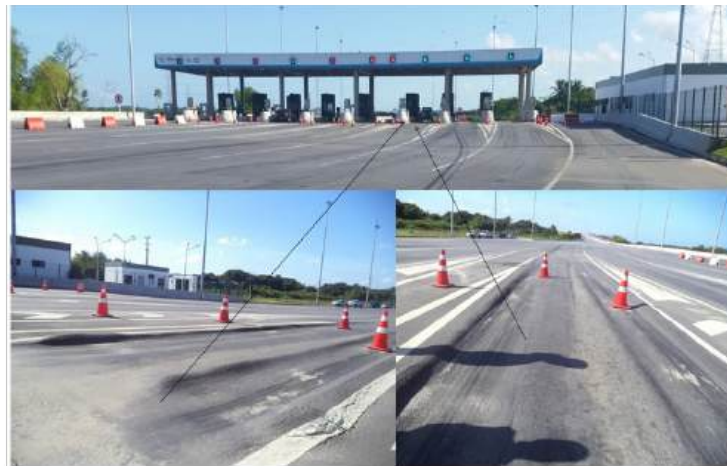
Figure 1 Plastic deformations of the asphalt mixture on the toll plaza pavement
