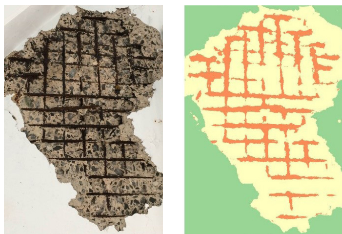
Fig. 2 Damage of segmentation results for the infrastructure
